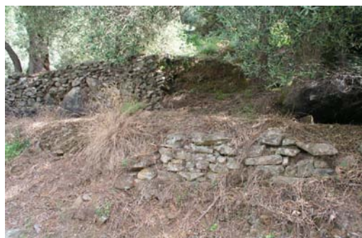
Figure 4. Lack of maintenance is evident in the dry stone walls
